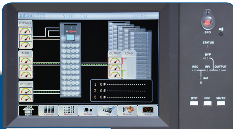
UPS FRONT PANEL
